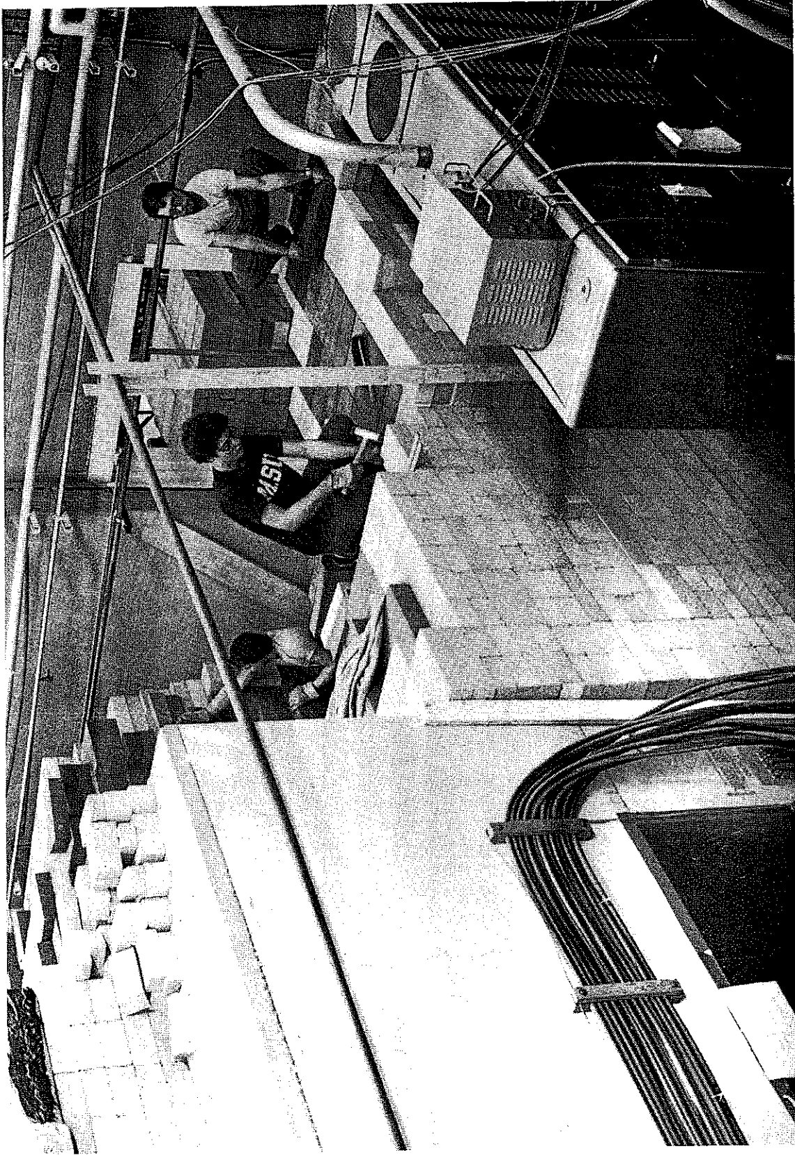
21. Fig. II. 20. Student workers in the process of reconfiguring the shielding wall for the Phase I beam transport system.
